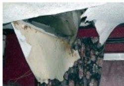
Collapsed ceiling, Birnies
