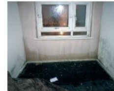
Soaked walls and floor, May Ct
