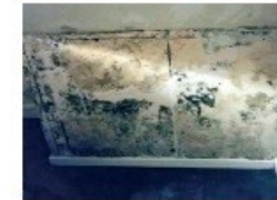
Damp and mould, Gunnet Ct.
